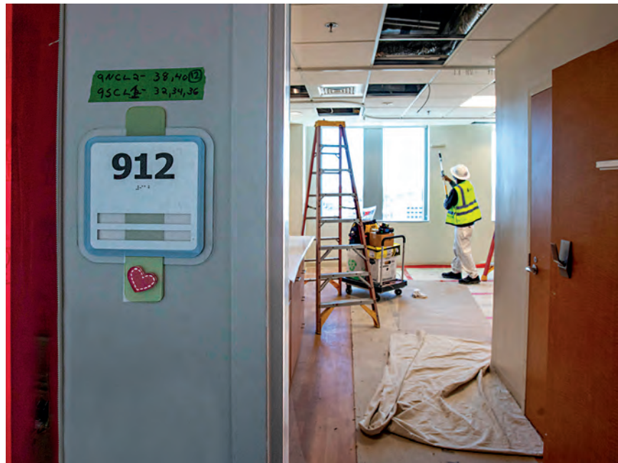
Le Bonheur Children's announced a major expansion in July 2021, including the 9th floor renovation pictured above. Construction is underway to expand critical care needs.
